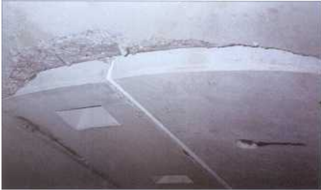
Damaged edges of a traditional reinforced segment.
