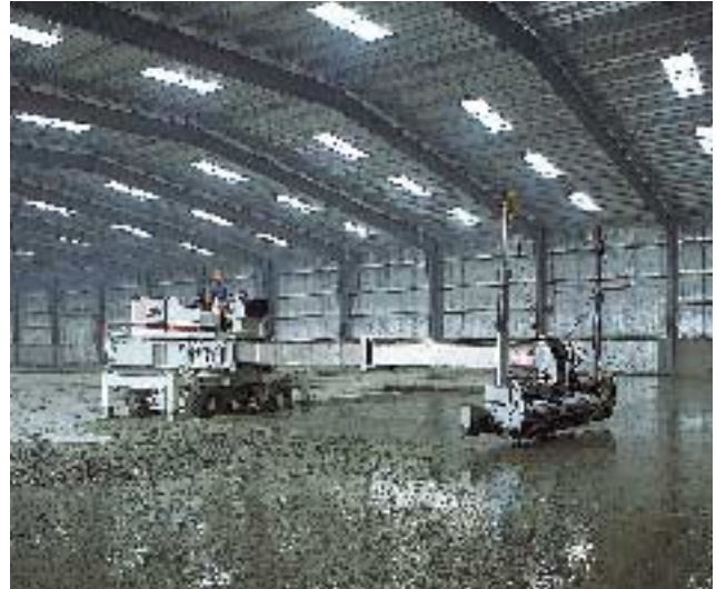
Forward to the present ... Modern placing techniques are labour efficient (laser screed, dumpers ...)
